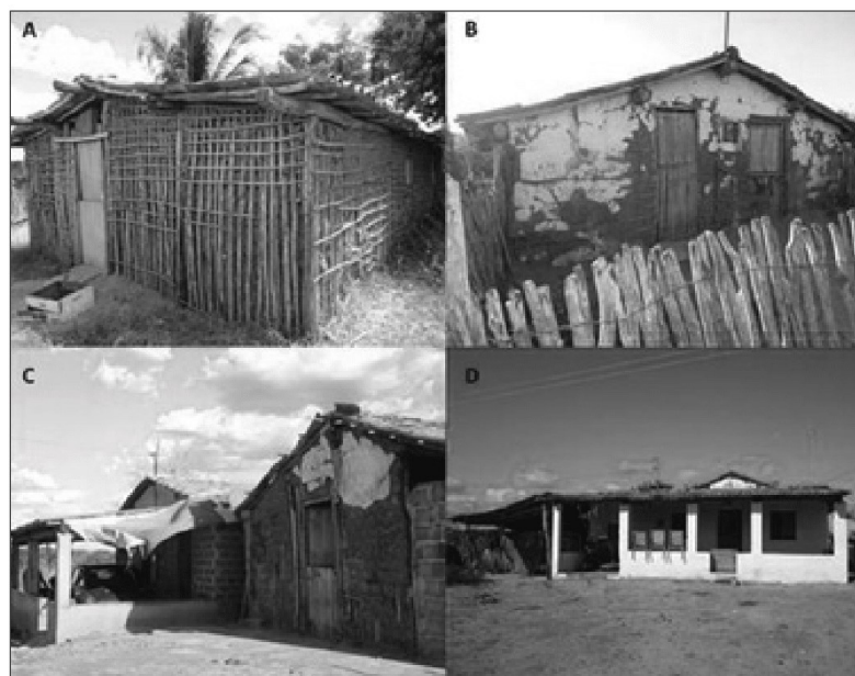
A A mud hut in which the outer surface of mud has collapsed, exposing the wooden frame. B A mud house partially damaged, although part of the coating of clay, painted white, is preserved. C A clay block house, newly built, beside a mud house.
